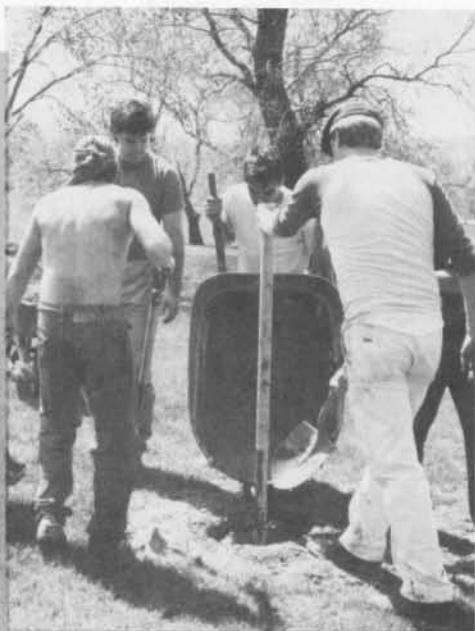
PFDS volunteers sweat out the last of the cement as Schenley Pole Holes are realized
